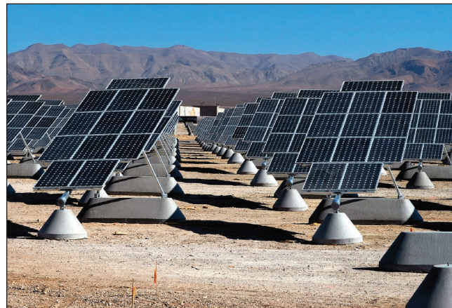
Figure 1.9 A power plant at Nellis Air Force Base utilizes photovoltaic solar cells. ©Stocktrek Images/Getty Images RF
